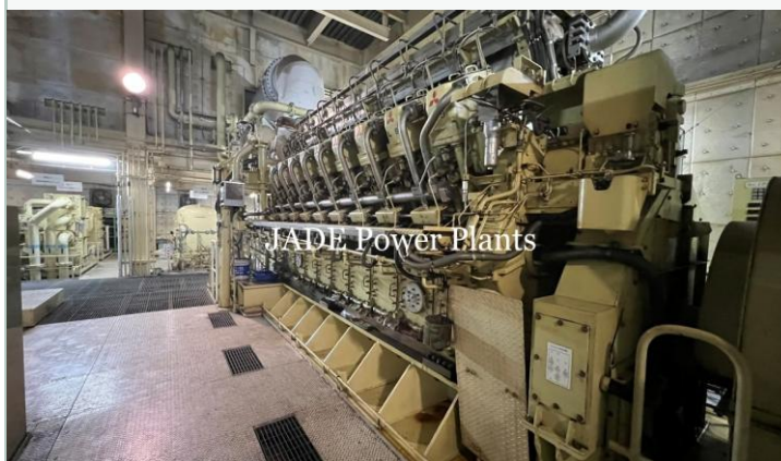
Mitsubishi 18KU30GA gas generating set
