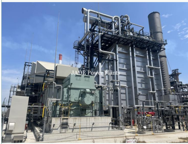
Kawasaki L30A gas turbine CHP plant
