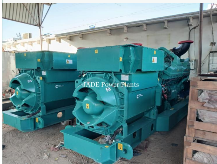
Cummins C2250D5 generator set
