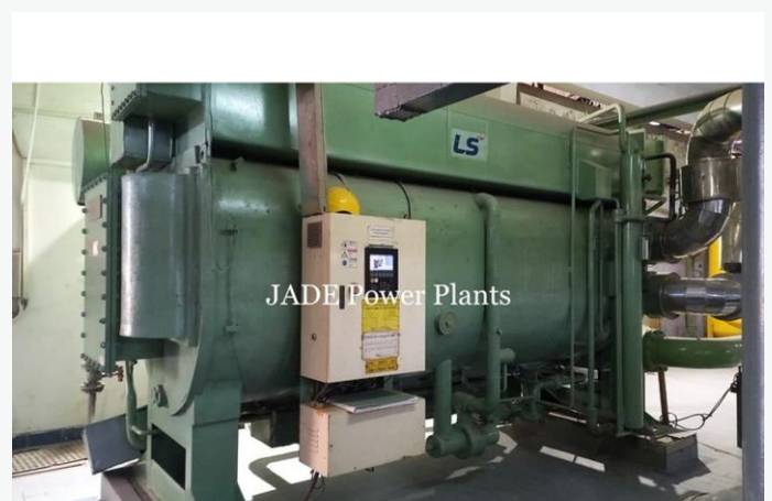
LS Double-Effect Absorption Chiller Actual plant photograph
