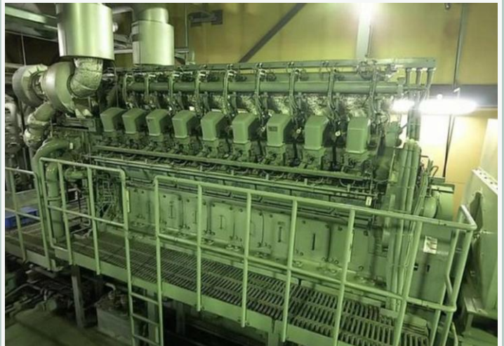
Niigata 18V22AG Gas Engine Representative Niigata 18V22AG Imagery
