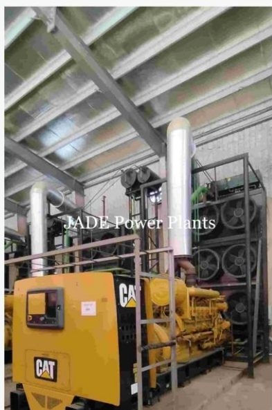
Representative CAT 3516B Control-Side View
