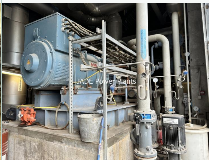
Steam Turbine Generator
