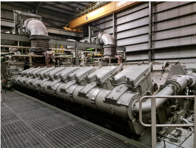
MAN 18V48/60 TS generating units
